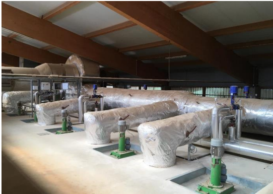
Figure 19: Piping for heating coils
