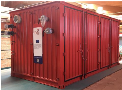
Figure 24: Heat Pump Container (outside)
