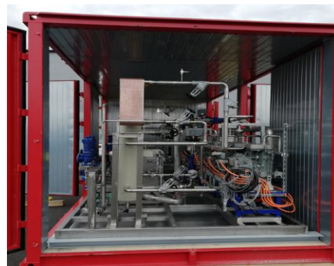
Figure 25: Heat Pump Container (inside)
