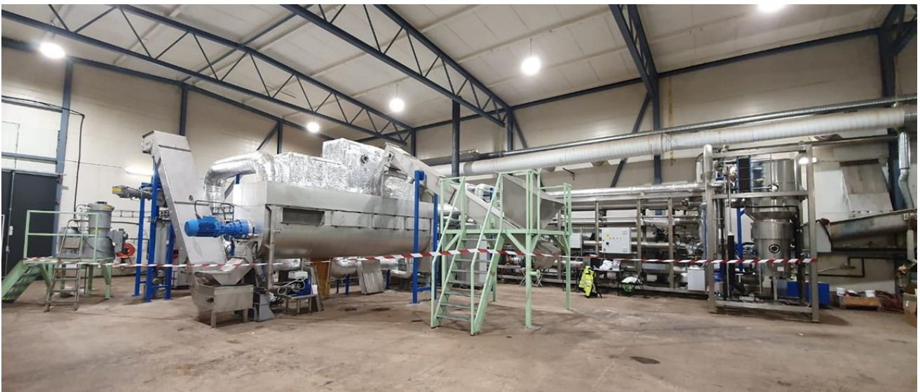
Figure 20 Complete SHS-dryer pilot (to the left) installation at Lindum with the open loop heat pump (in the back to the right).
