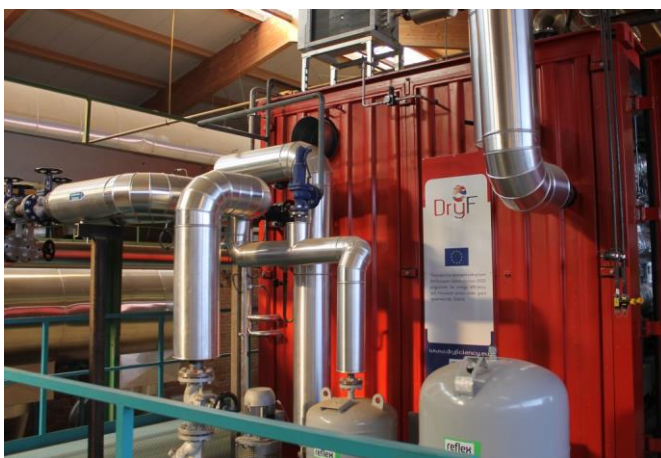
First industrial high-temperature heat pump at Wienerberger Österreich GmbH at the Uttendorf site in Upper Austria in demo operation © AIT / Schneeberger
