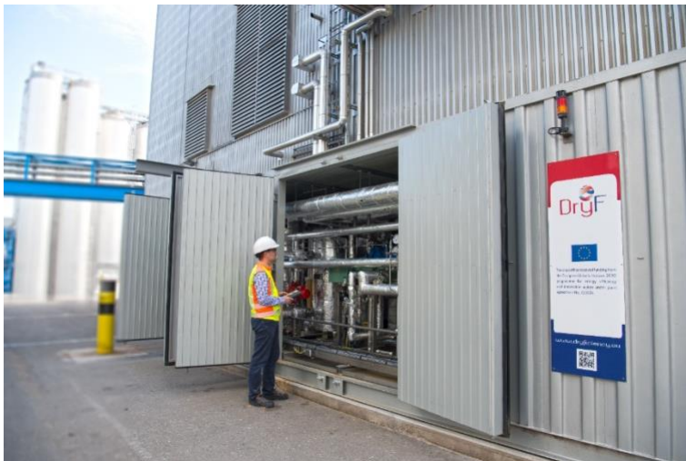
BU: DryFiciency high-temperature heat pumps were commissioned in three applications and tested in an industrial environment. Plant at AGRANA Stärke in Pischelsdorf. © AGRANA
