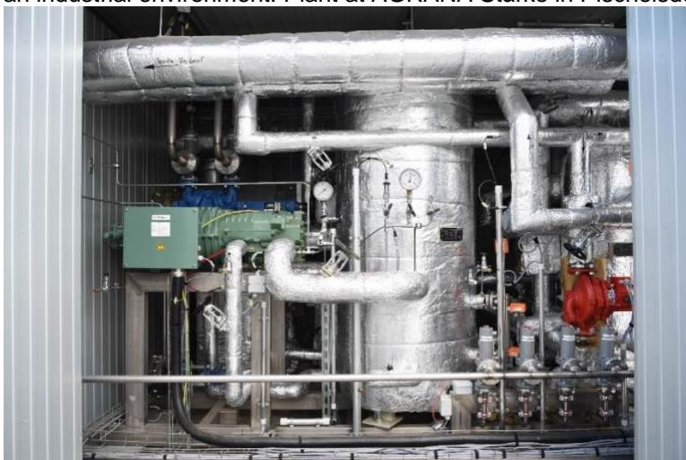
BU: DryFiciency high-temperature heat pumps were commissioned in three applications and tested in an industrial environment. Plant at AGRANA Stärke in Pischelsdorf. © AGRANA
